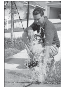
Fixing broken sprinkler heads is an easy way to conserve water.
