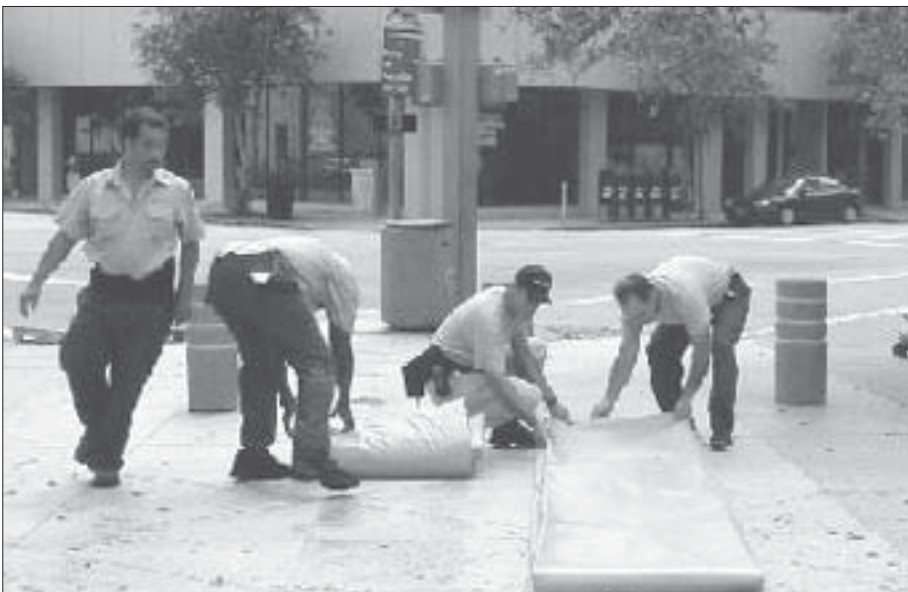
Facilities Management employees prepare the water barrier that was placed around the County Center before Hurricane Ivan. It took staff four hours to prepare the flood barrier.
