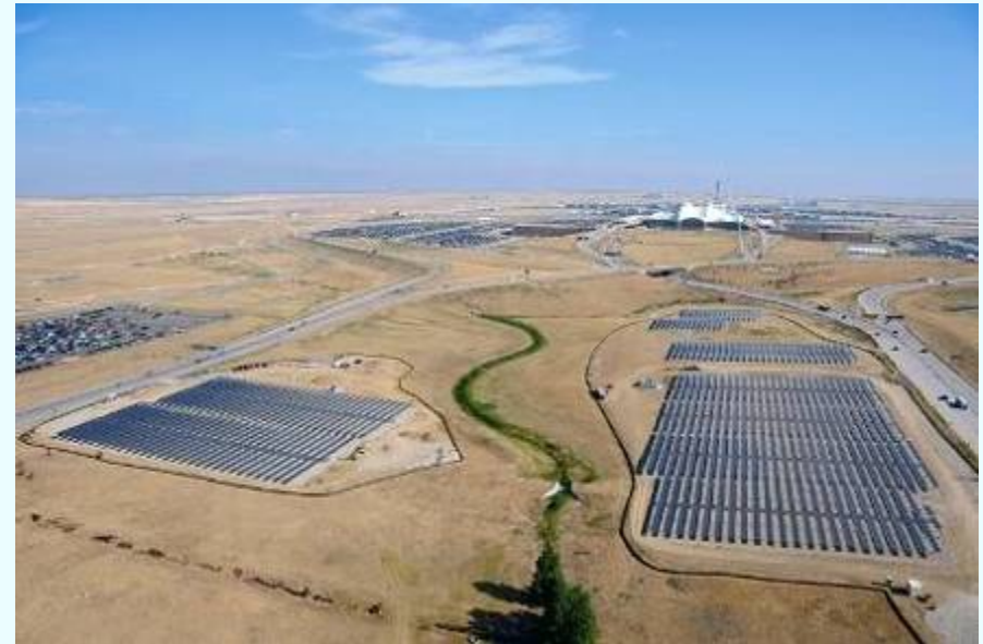
Denver International's 2 mega-watt solar array
