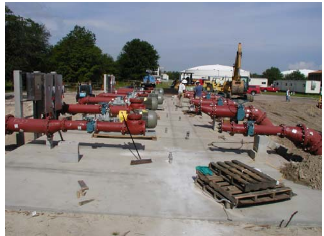
Lithia Pinecrest RW Storage and Pumping Station
