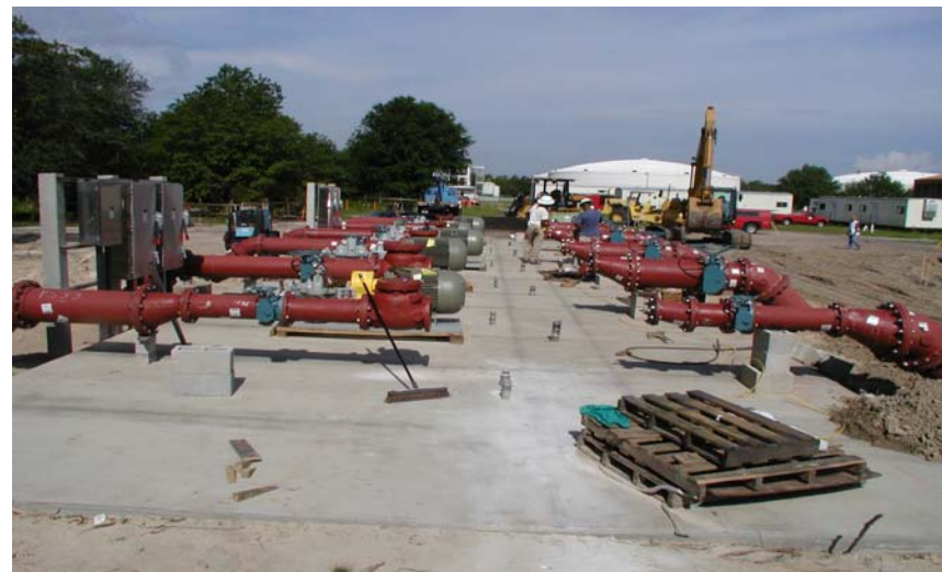
Lithia Pinecrest RW Storage and Pumping Station
