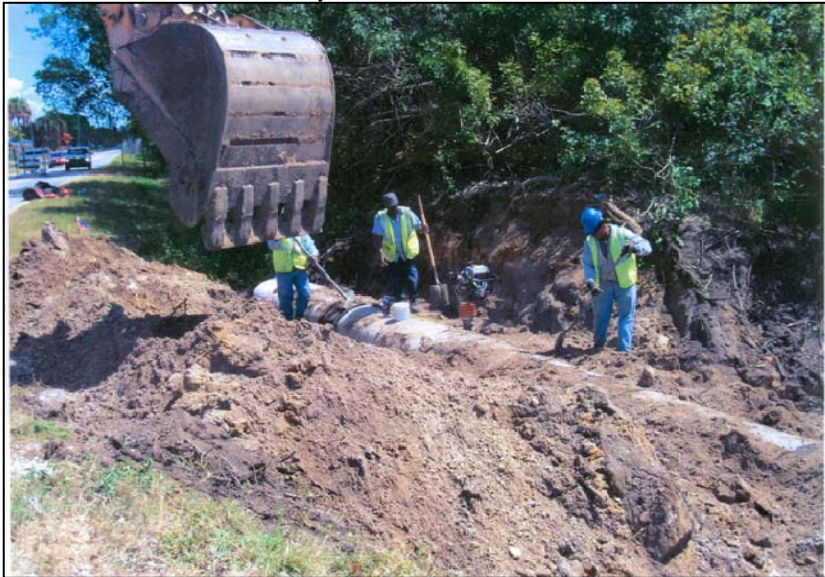
Stormwater improvement projects such as this will alleviate flooding in the unincorporated area of Hillsborough County.
