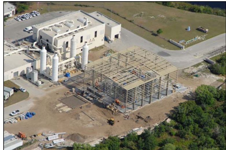
Northwest Class A Sludge Processing Facility
