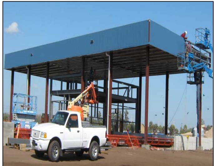
Construction of this entrance canopy is just one of many improvements being made to the South County Transfer Station.
