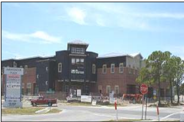
The Town n' Country Commons complex, housing the Town 'n Country Library, is currently under construction.
