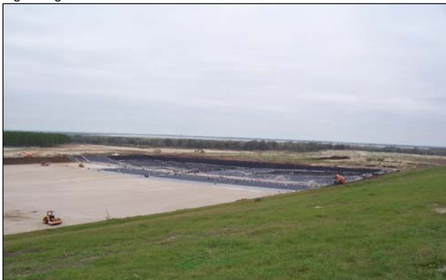
The Southeast Landfill Capacity Expansion project will add capacity for future County customers.
