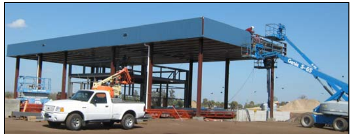
Construction of this entrance canopy is just one of many improvements being made to the South County Transfer Station.
